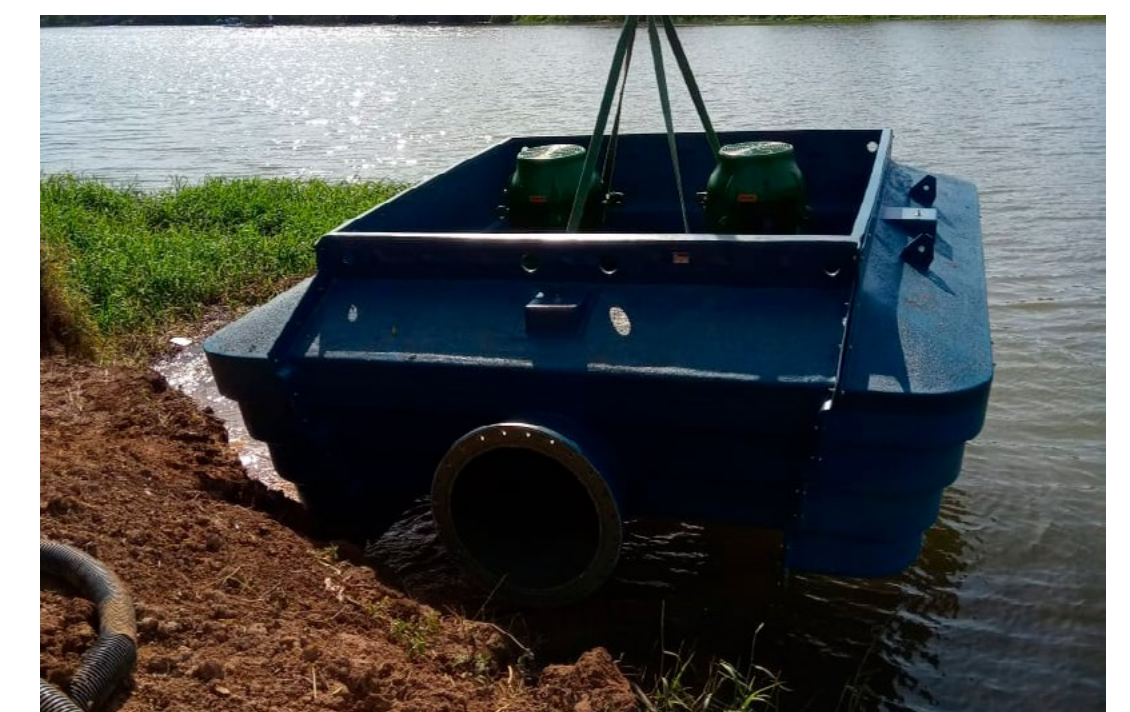
Reverse station pump floater/buoy
