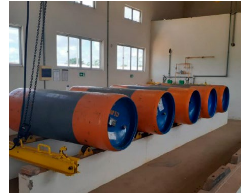
Old chlorine gas system
