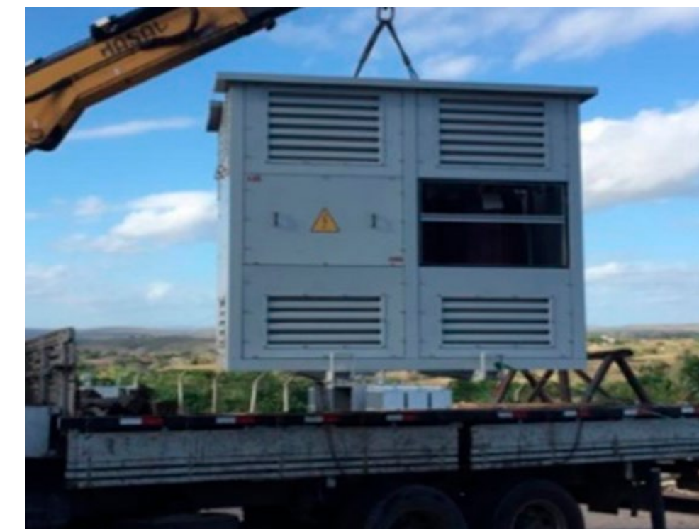
New transformer of the TWPS (Treated Water Pumping Station) 02
