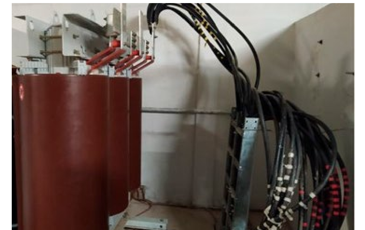
New Transformer of collection Traipu
