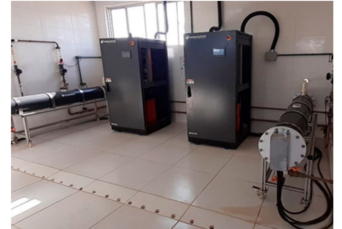
New hypochlorite generator system
